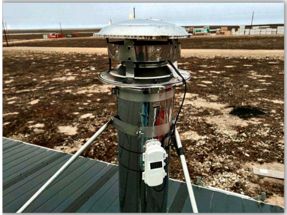
Fig. 1. Temperature/humidity sensor on boiler and water heater exhaust stack
